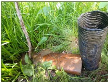
8-inch pipe draining source water for wetland and vernal pool complex.
